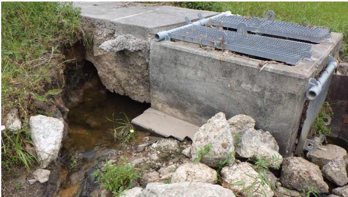
Figure 5. Bank collapse at water diversion structure.
