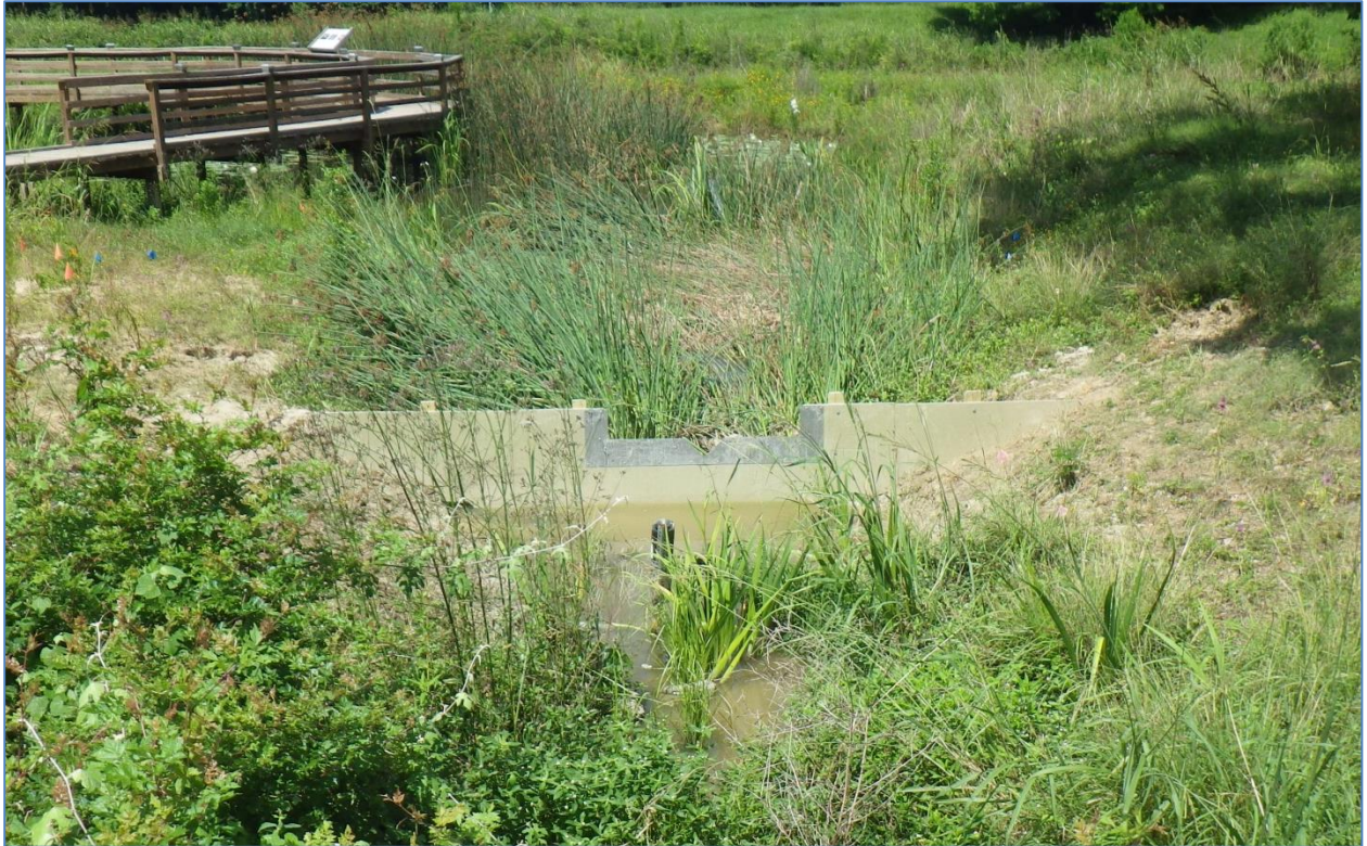
Figure 11. V-notched weir installed at the most upstream point of the secondary wetland, UHCL created wetland site. The weir is used to monitor water flow.
