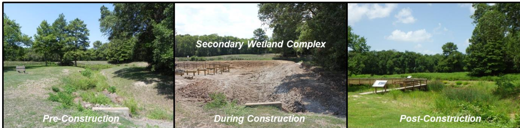
Figure 13. Time-series photographs of the secondary wetland complex showing pre-construction, during construction, and post-construction conditions.
