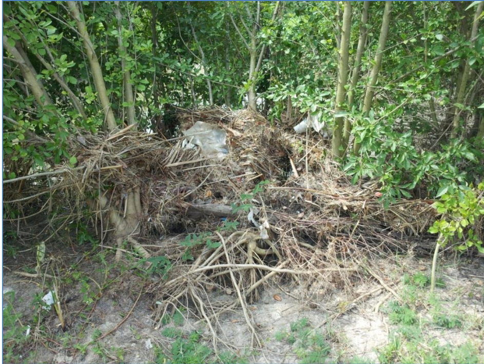
Figure 14. Accumulated debris at the edge of pond 3 observed on June 31, 2012 believed to have been deposited by recent flood events.
