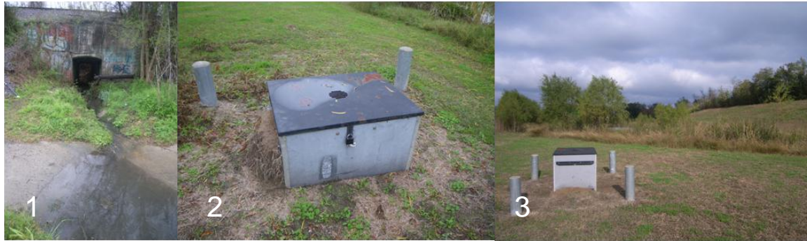
Figure 6. Mason Park field survey site photographs (1 – inlet to wet pond; 2 – North Agridrain box; 3 – South Agridrain box).
