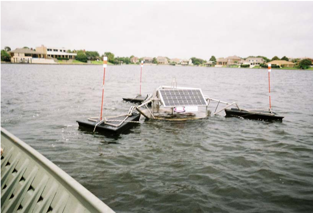
Figure 4. Solar powered aerator assembly floating in middle of Lake Madeline.
